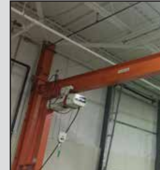
HALF TON JIB CRANE WITH HOIST
