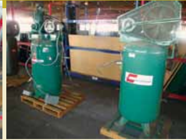
(2 OF 3) VERTICAL AIR COMPRESSORS
