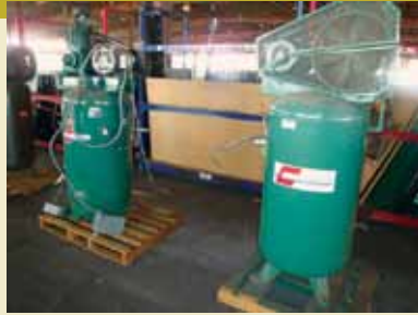
(2 OF 3) VERTICAL AIR COMPRESSORS
