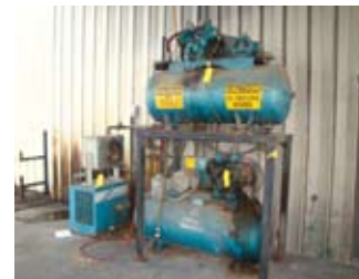
(2) KELLOGG AIR COMPRESSORS
