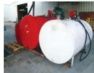
VARIOUS FUEL TANKS
