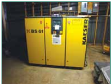
KAESER 25 HP AIR COMPRESSOR
