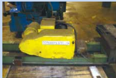
(2) Overhead Cranes With Crane Rails, 5 Ton Gantrys, And Cable Hoists
