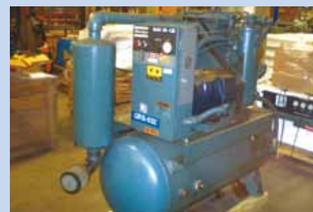
Atlas Copco Air compressor
