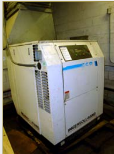
INGERSOL RAND 40HP AIR COMPRESSOR
