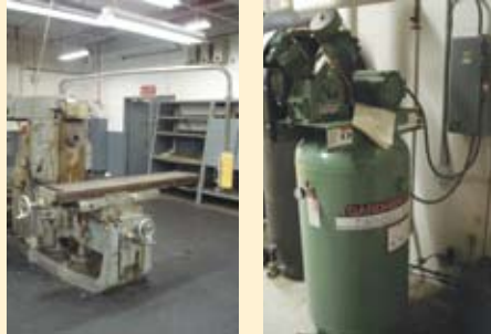
LEFT: FREZARKI Universal Mill RIGHT: GARDNER DENVER Vertical Air Compressor
