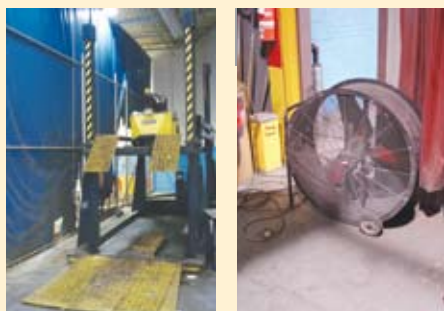
LEFT: Lift-A-Lift Fork Truck Lift Station (30,000 Lb. Cap.) RIGHT: Huge Qty. Of Floor Fans
