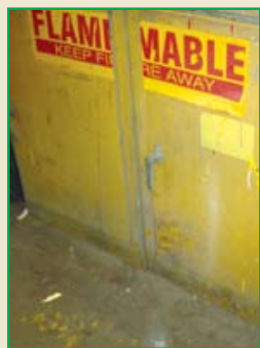
VARIOUS FLAMMABLE LIQUID STORAGE CABINETS
