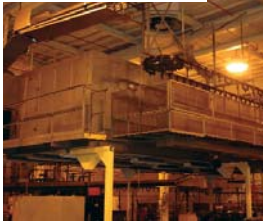
COMPLETE ELECTROSTATIC PAINT SYSTEM
