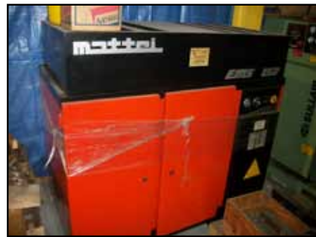
MATTEI ROTARY SCREW AIR COMPRESSOR
