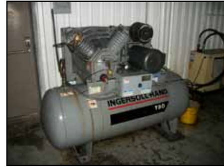
INGERSOLL RAND T30 AIR COMPRESSOR
