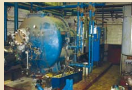
INGERSOLL RAND 900 HP AIR COMPRESSOR
