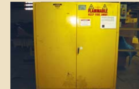
VARIOUS FLAMMABLE LIQUID STORAGE CABINETS
