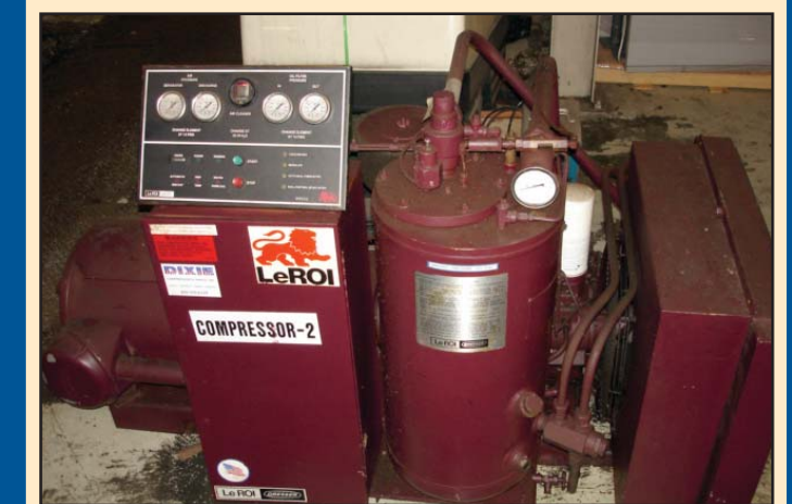
(1) OF (3) LEROI ROTARY SCREW AIR COMPRESSORS
