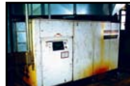
INGERSOLL RAND 150 HP AIR COMPRESSOR
