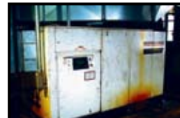
INGERSOLL RAND 150 HP AIR COMPRESSOR
