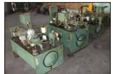
OIL CIRCULATING TANKS
