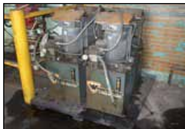
COOLANT CIRCULATING PUMPS
