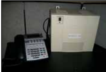
NEC PHONE SYSTEM (4) TELEPHONES AND (1) ELECTRA ELITE 48 BASE STATION
