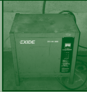
(1 OF 4) VARIOUS BATTERY CHARGERS
