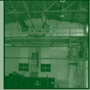
6-TON OVERHEAD GANTRY CRANE
